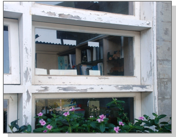
Peeling paint around a window: soon to be history!
